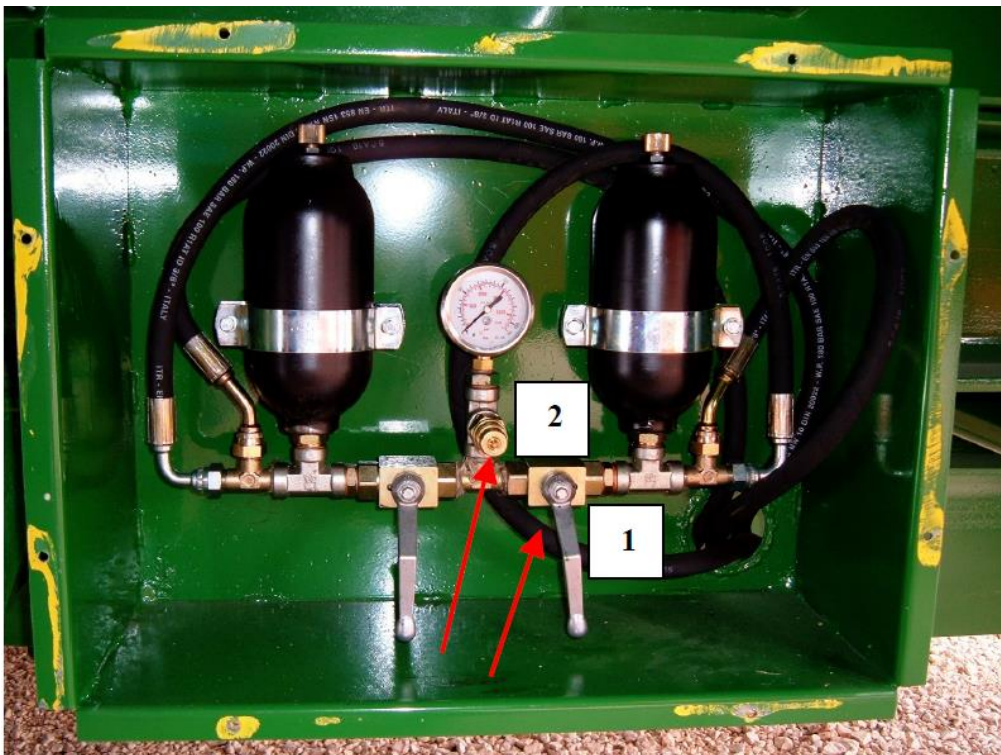
Figure 8 Connecting Point setup on a Tandem axle trailer with one passive steer axle
