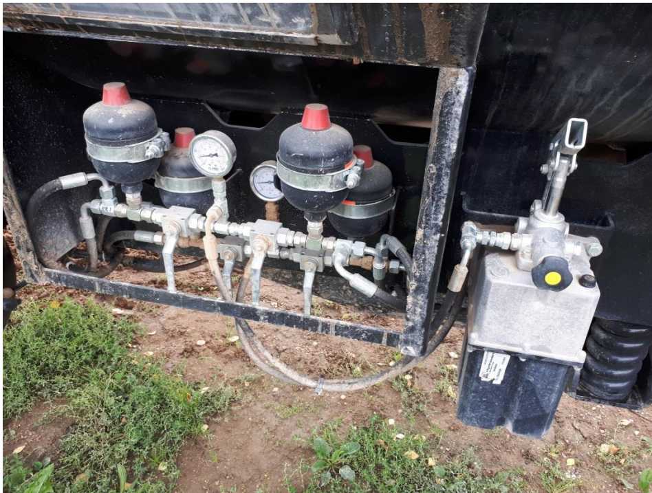
Figure 4 Example of Tri-Axle Gas Accumulator + Pressure Gauge + Hand Pump setup
